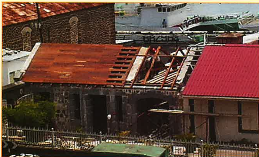
The Conservation Work on the Hospital Block at the Aapravasi Ghat in October 2005
